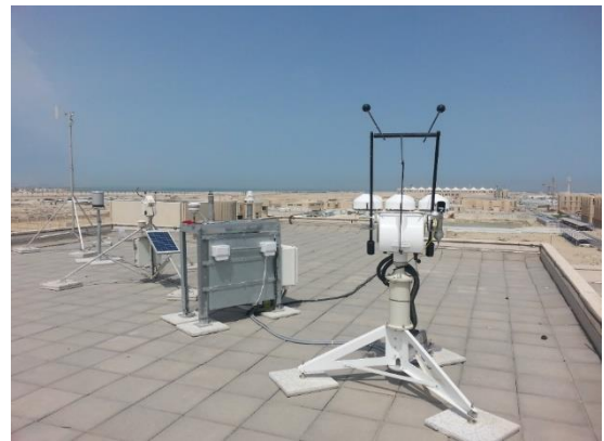
Figure 5. Solar monitoring station at the roof top of the College of Architecture & Planning
